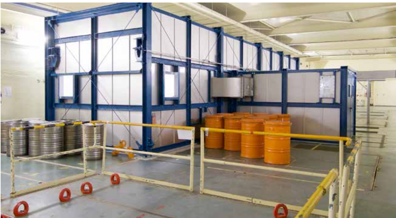
View of the hatch for bringing in and removing material (front) and of the dismantling caisson in the crane hall above the cells.
