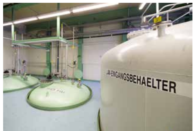
Chemical effluents and other unburnable liquids are sampled in large tanks and reduced in volume by evaporation.
