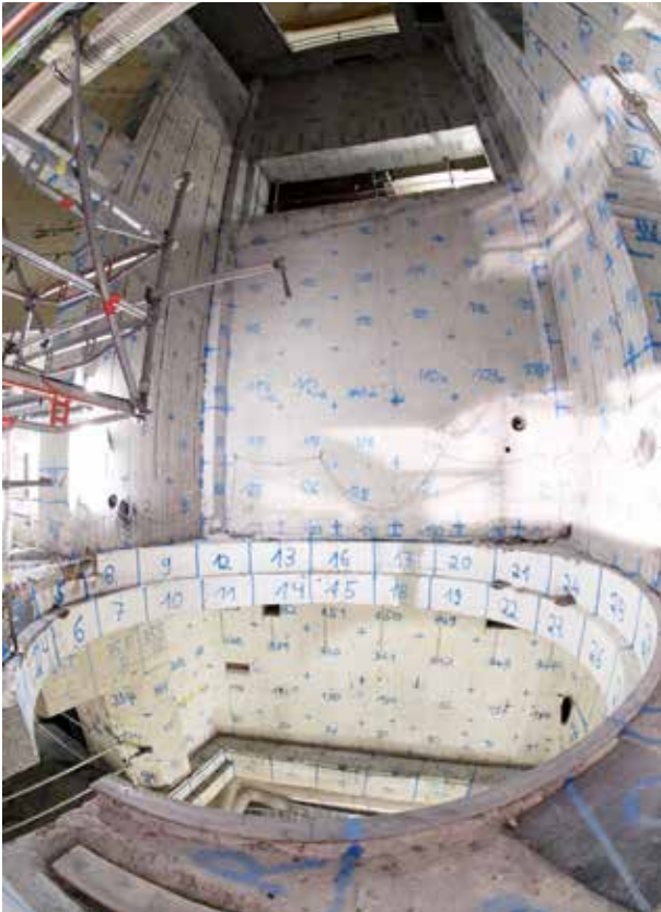
The end of the project is near. Now, the main tasks are measuring, reworking, measuring, controlling, and confirming.
